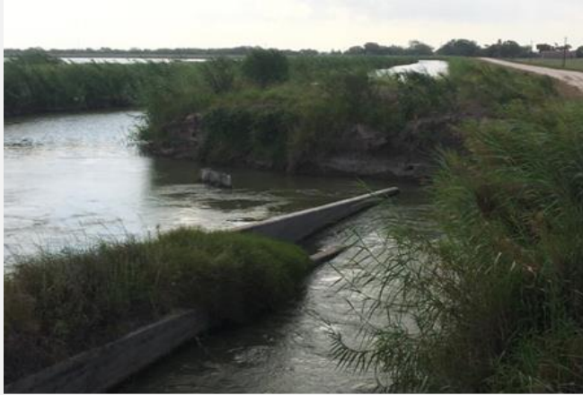
Existing Mercedes Levee Gap Failed Structure
